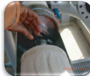
UNIT 3 is installed and connected to the permeate collection tube of the existing vessel using all existing hardware.
