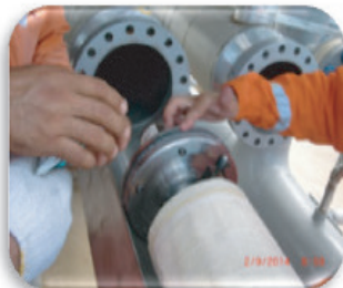
UNIT 1 is pushed into the existing vessel along with the residue side seal assembly attached.
